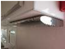
Vented exhaust fans
